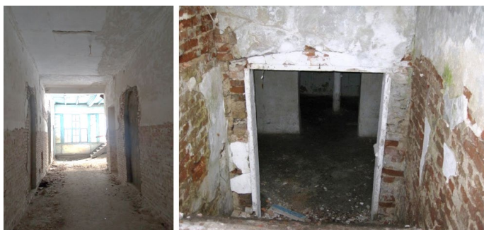
Figure 7, 8. The mansion of the Polish boyar Ohanowicz – the interior space on the ground floor and the staircase leading to the basement [25]
